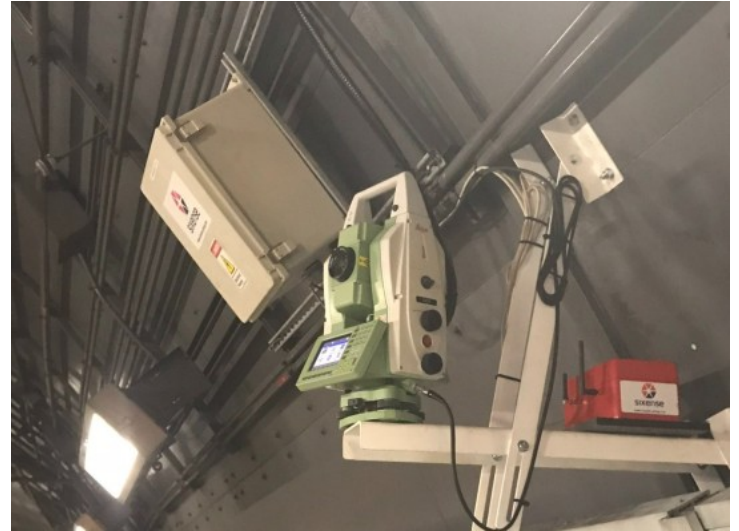
AMTS and Vibration Installation
